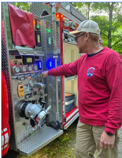
Chief Phil Severy at the pump panel of Rescue One adjusting water pressure.
