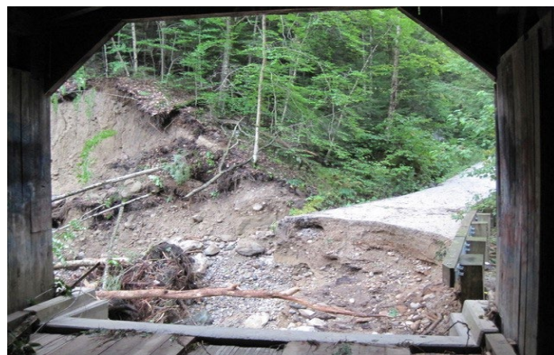
Scour visible from Brown Covered Bridge after Irene
