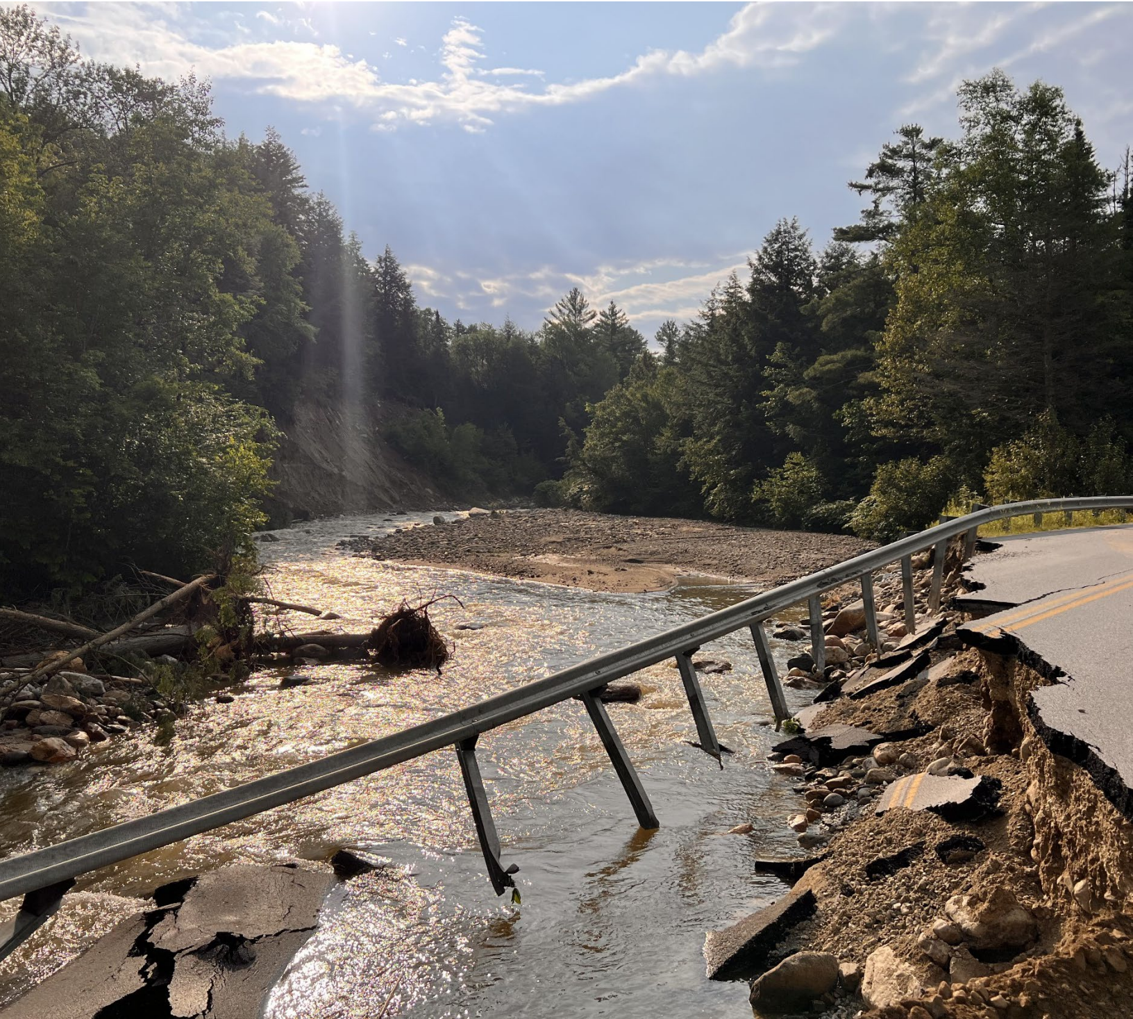
Cold River Road undercut by a dynamic shift in the river channel – July 2023 (DR4720)
